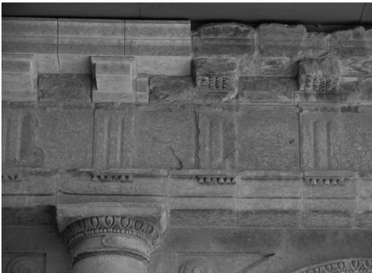
Fig. 9. Detail of the moldings consolidation execution, performed in 2009, on the entablature of the area projected by Juan de Herrera in the cloister of the Cathedral.
